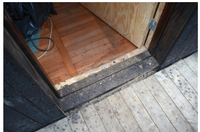
Threshold almost at the same level as the deck makes it easy to enter.
