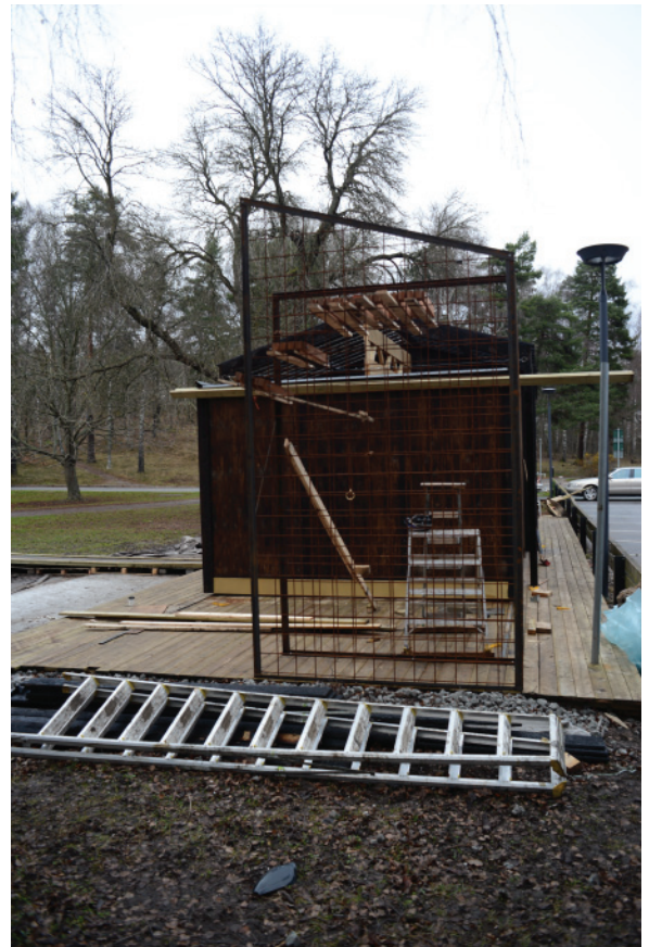
Staircase in construction to access the roof of the Friggebod. This is where the deck is almost at the same level as the ground. The entrance could have been located here to make the hole deck more accessible.
