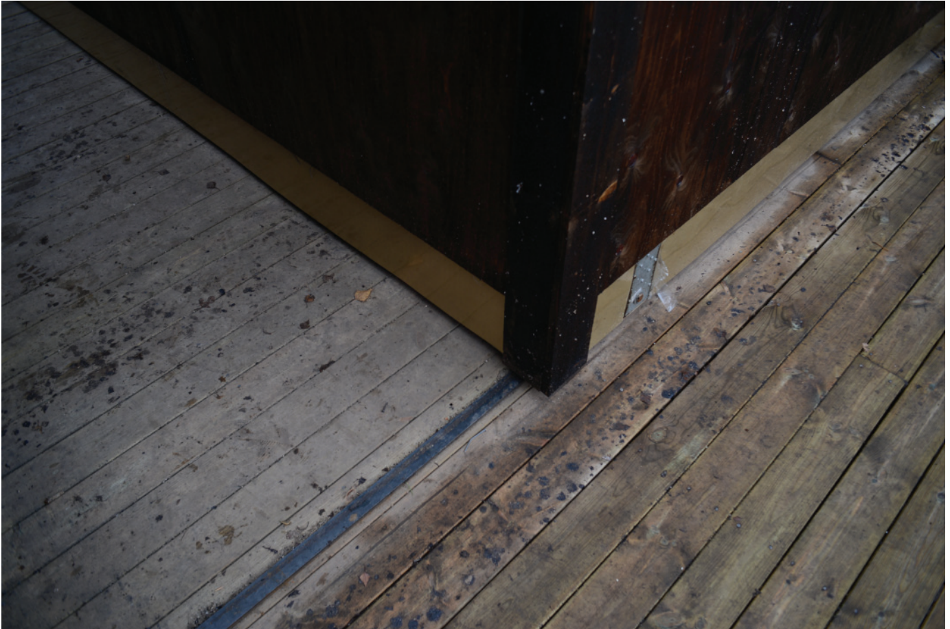
The rails in the deck is for the Friggebod to slide on. Dirt and leaves has been collecting on the inside of the rail, therefore it is hard to sweep the deck clean with a broom.
