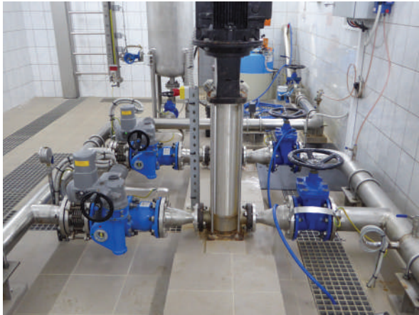
Photo 5: The pumping room
