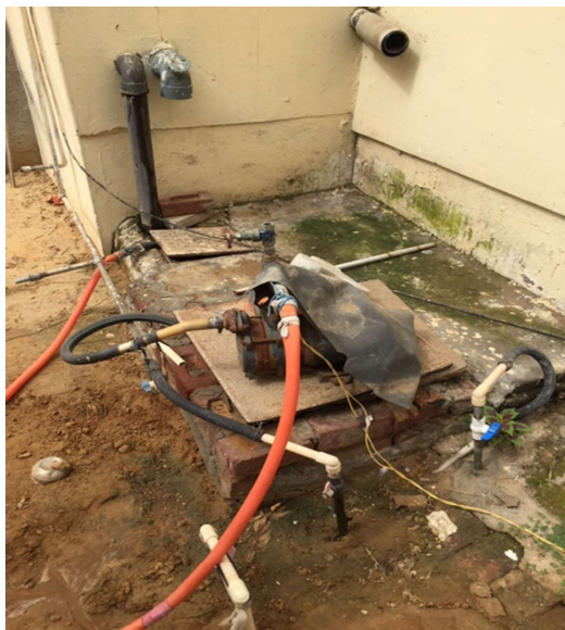
Figure 3: Pipes and pumps to lift water supplied by DJB to higher floors in a private bungalow
