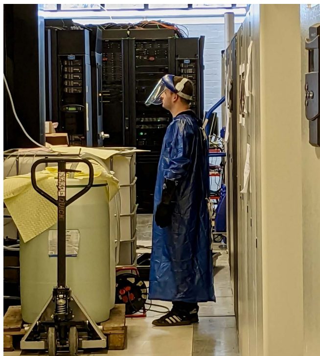
Above: An HPE technician wearing protective gear while overseeing the process of changing the cooling water
