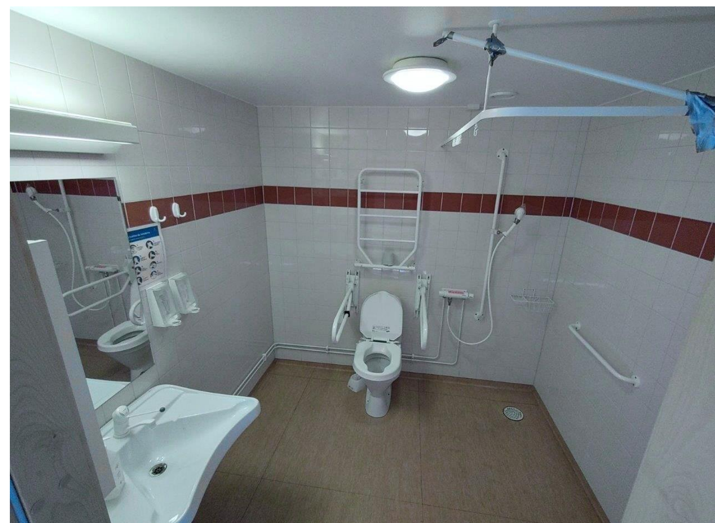
Bathroom 1 "Nursing home" was a large nursing home bathroom equipped with standard assistive devices.
