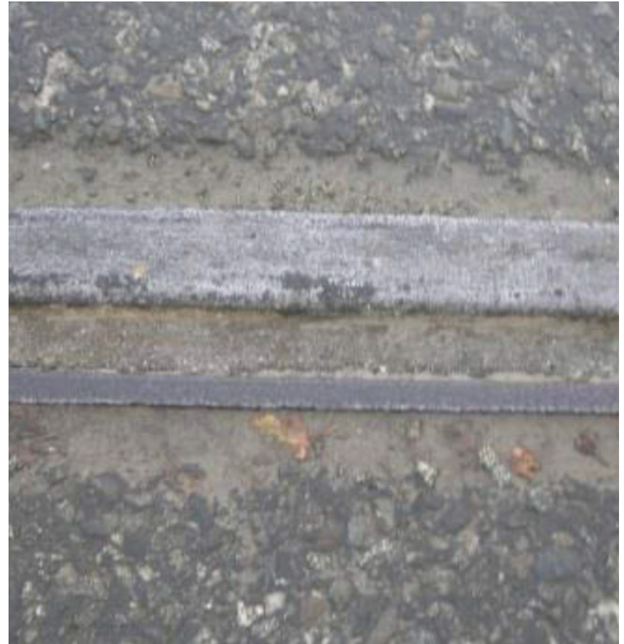
Dark coating forming when \text{MgCl}_2 is drying
