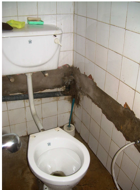
Plate No. 4 : WC fitted by Tenant at Ubungo Block H(2007 Photo) -
