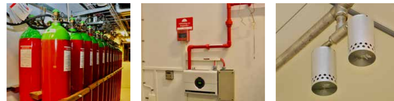
Above: (left) Rack of high-pressure gas bottles containing Argonite to suppress fire breakouts (centre) The sampling smoke detector sucks in air from the red pipe which has small holes at regular intervals and uses a laser detector to measure the smoke level in the room. (right) The nozzles where the gas enters the room are equipped with silencers to reduce the sound level when the gas is released. This is important as modern hard disks are sensitive to (and could be damaged by) high sound levels.
