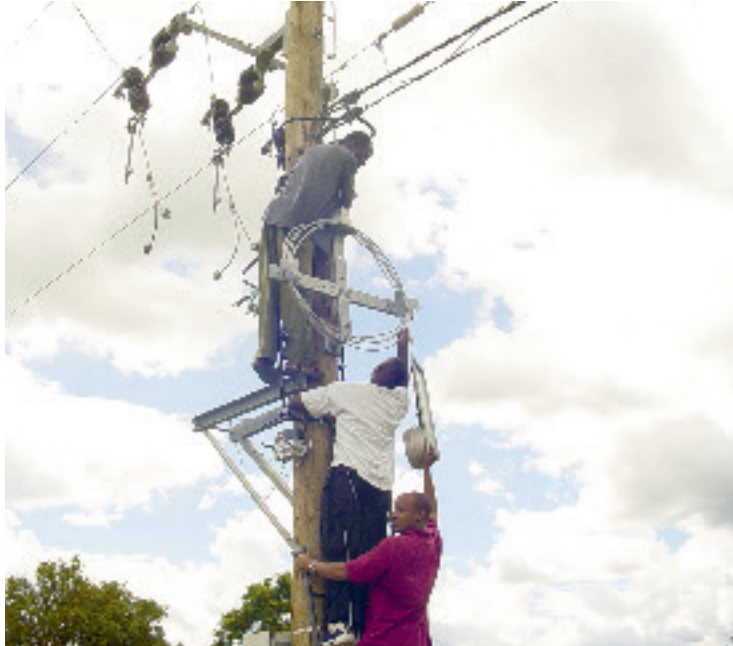
Installation of solar-powered router in Tanzania, Photo: Björn Pehrson
