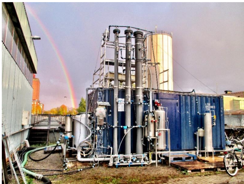
Figure 4. Mobile pilot plant for removal of pharmaceutical residues from effluent of waste-water treatment facilities.
