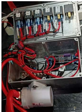
(a) Relay box
