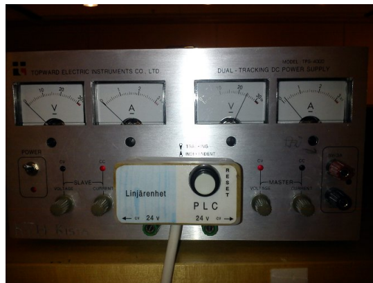
Figure 6: PLC power connected to DC power supply
