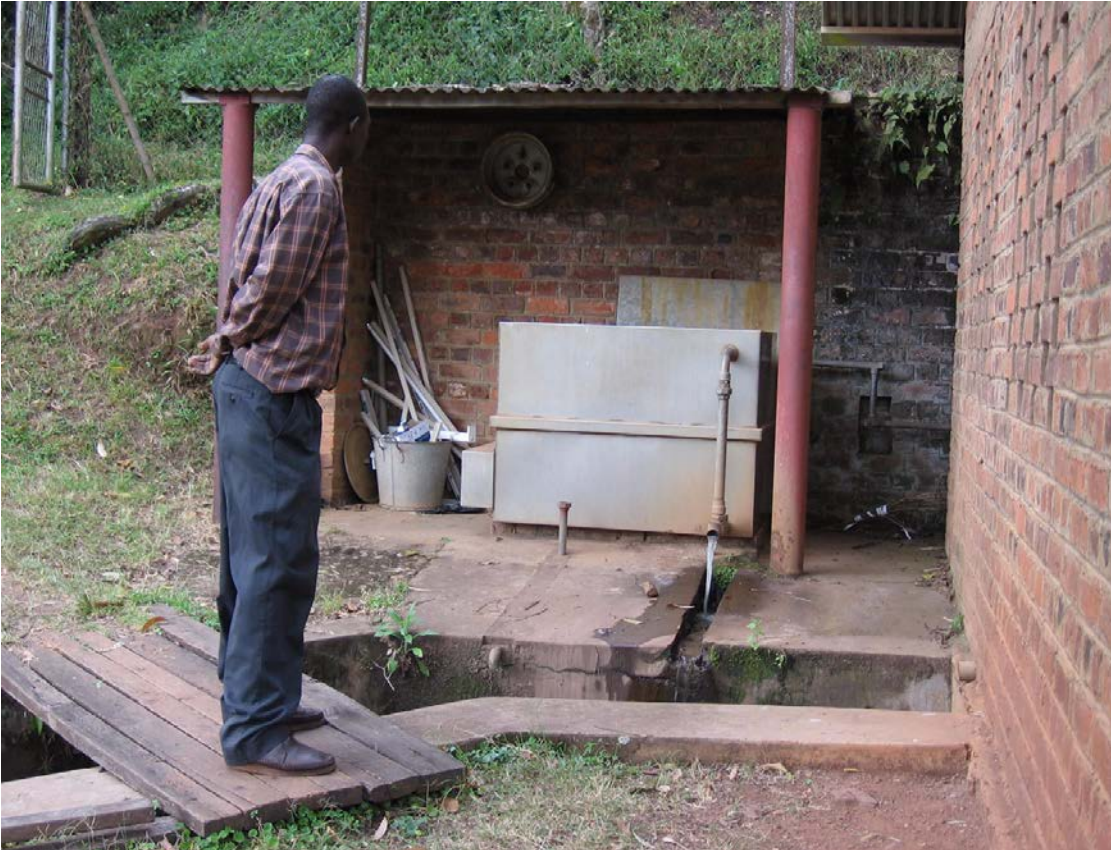
Kisiizi Hydro Power Plant, Uganda
