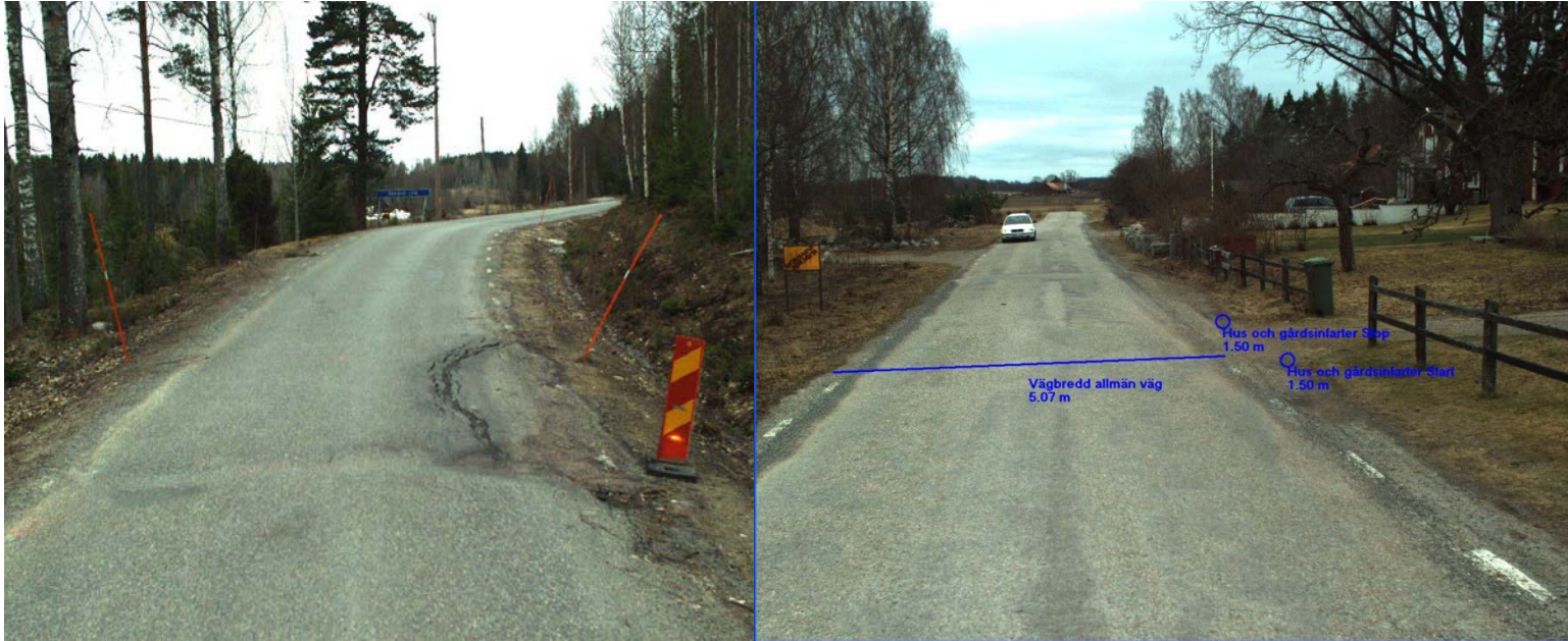
Inspection of damages
