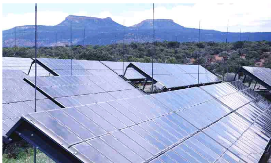
Solar panels used for power production.
